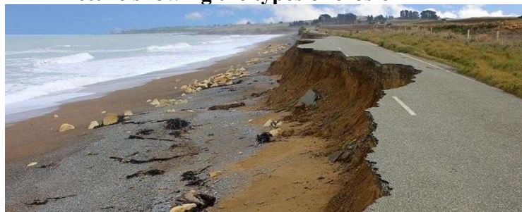
Picture showing soil erosion
